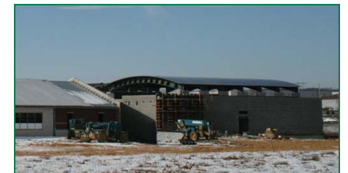
Jaindl Elementary School Breinigsville, PA PCMA Producer - New Holland Concrete LEED for Schools 2.0
